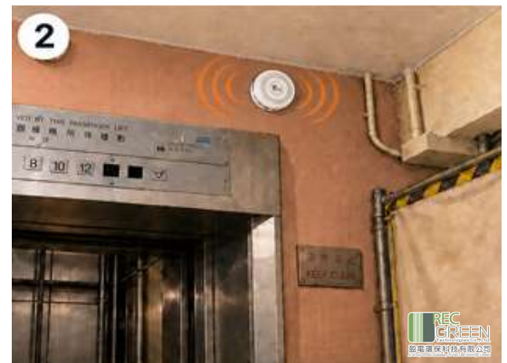
2 Detector immediately triggers an on-site alert and send the message to the platform
